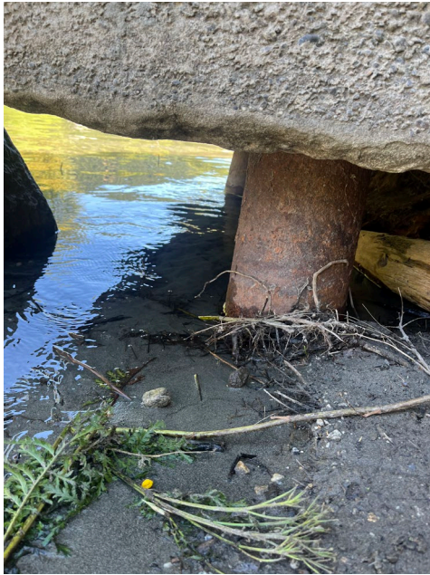
Scoured pile cap on the western abutment of the bridge.
